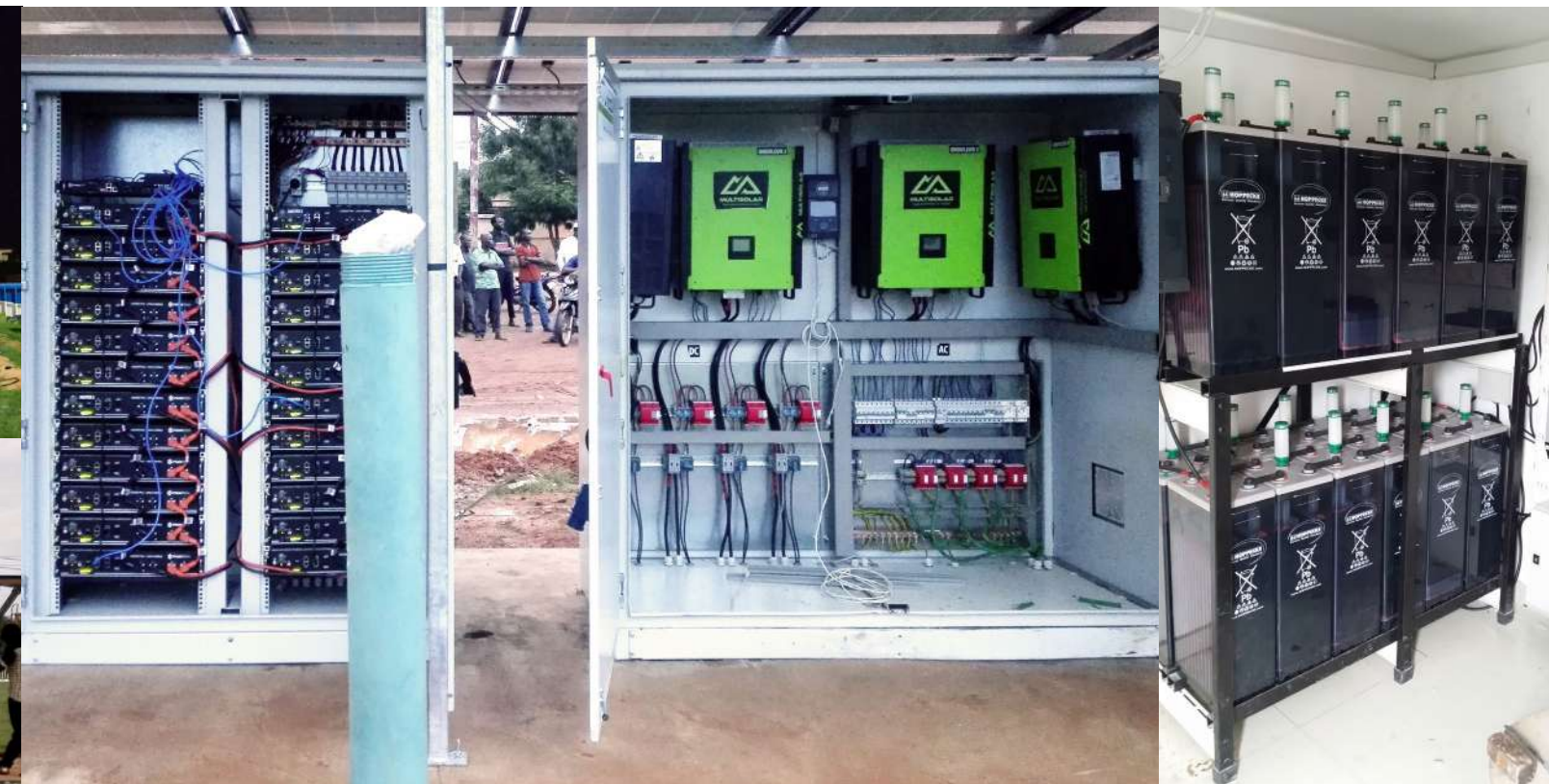
Installation of battery banks.
